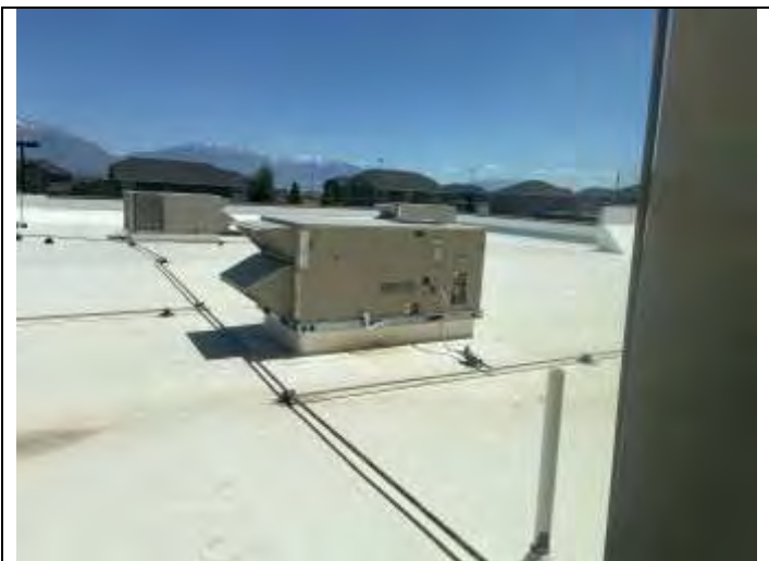
57. Roof-top HVAC equipment.
