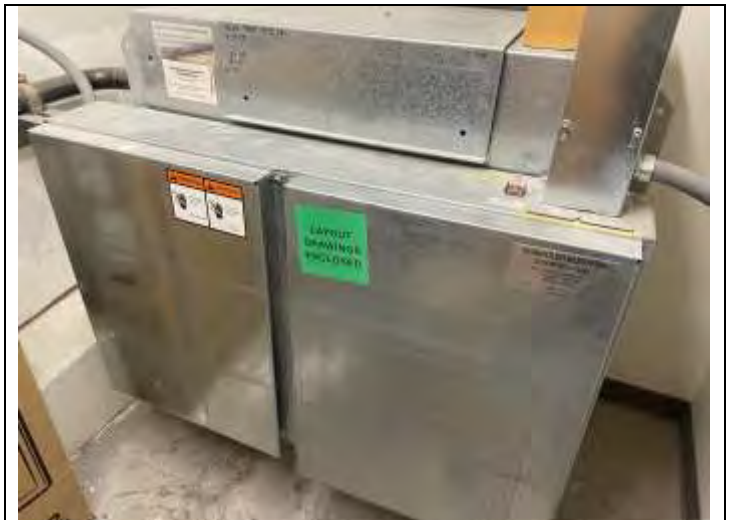
46. Hydraulic elevator equipment.
